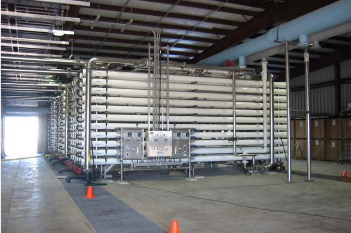
Southmost Regional Water Authority Reverse Osmosis Facility, Brownsville, Texas (photograph from NRS Consultants report by Joseph W. Norris).
